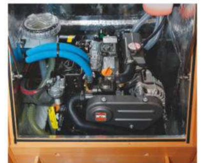
Engine access is okay but access to oil filters and the impeller cover is limited
